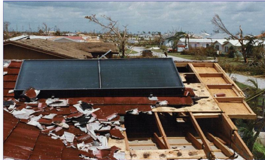
Panels on hurricane damaged roof in Florida. From One Block off the Grid: http://1bog.org/yes-solar-panels-can-survive-a-hurricane/
